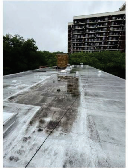
The darker area on this rectory roof shows where the water is pooling and seeping down through the ceiling of the rectory. We are currently addressing this issue before addressing the water damage inside the building.
