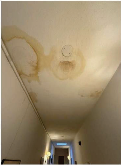
Along the second floor hallway, you will find many areas where water has come through from the roof just like this. It is even worse inside Fr. Abraham's rooms.
